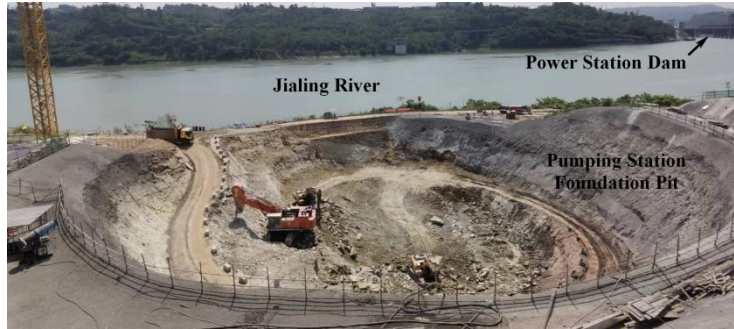
Fig.1 Real scene of pumping station
